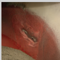
Position in need of repair
