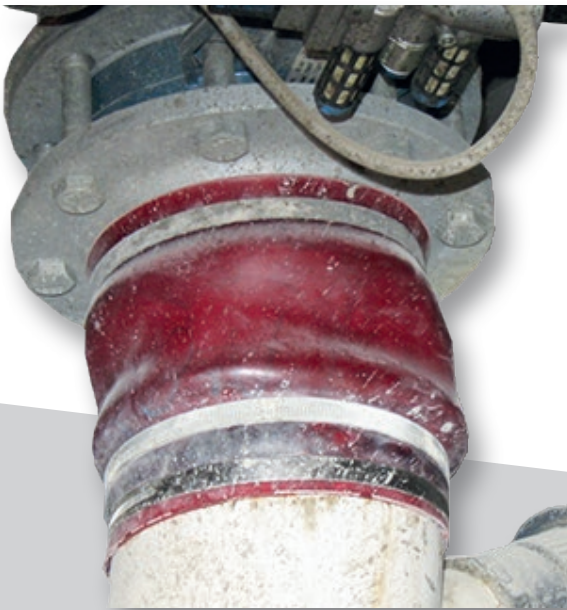
transfer sleeve water level / mixer
